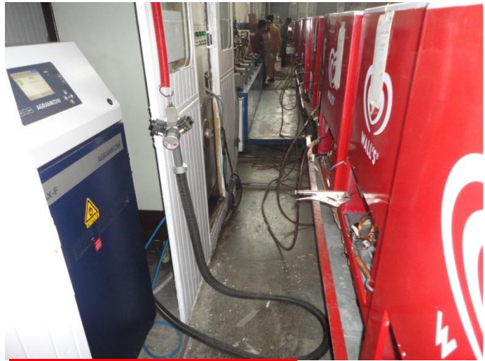
SARA-MAX-F CHARGING STATION
