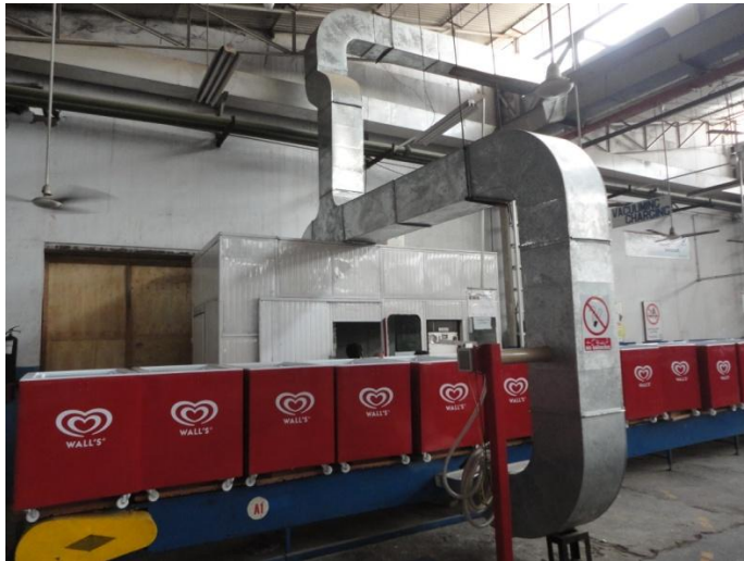
BLOW OFF UNIT AND VENTILATION DUCT.
