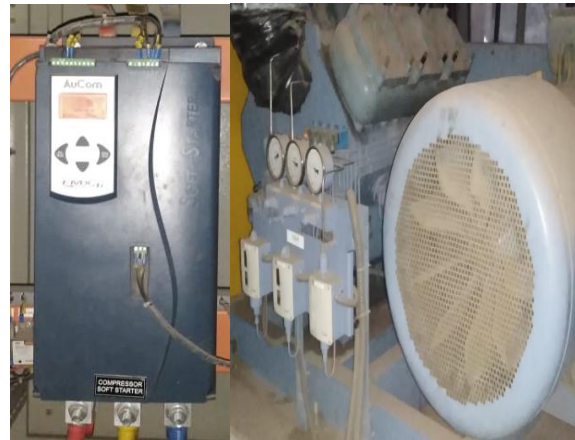
Fig 5: AuCom Soft starter, Compressor with Danfoss Pressure Switches.
