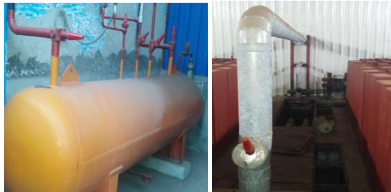
Fig 4: shut-off valve / regulating valve / check valve / check & stop valve / strainer valves/ Sovs/Sensors etc. fitted on discharge and return lines of R-717.
